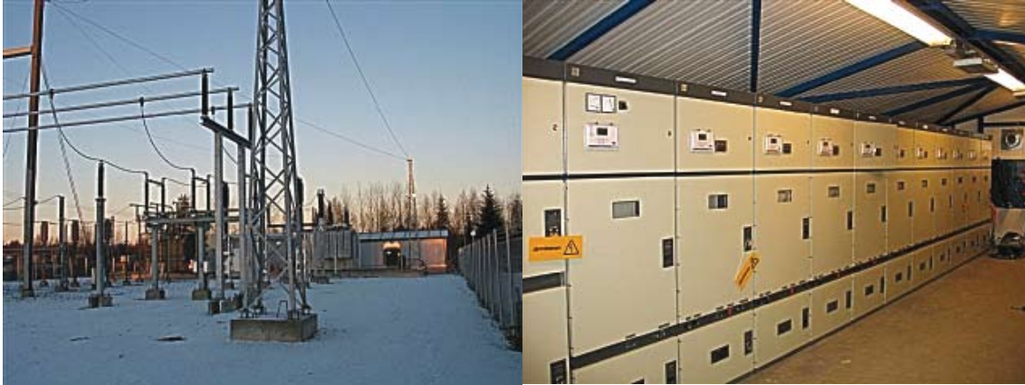
The Oulunsalo substation is equipped with 13 Vamp 255 protection relays.
